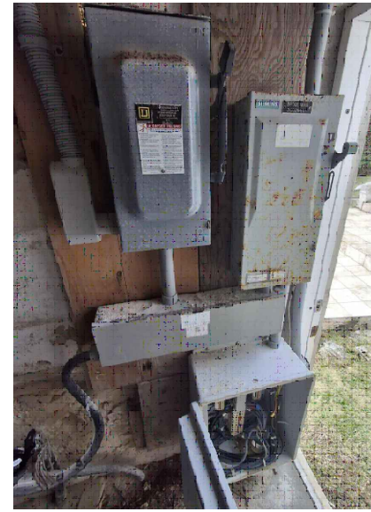
EXISTING BRIDE DISCONNECT AND CONTROL WIRING
